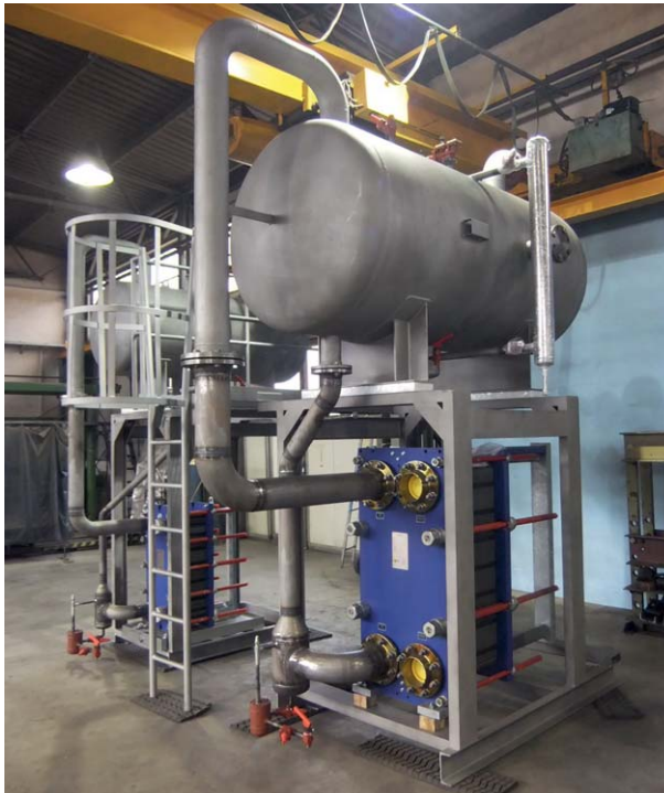
Figure 4.12 Liquid separator (also known as surge drum) (© EM Polar)
